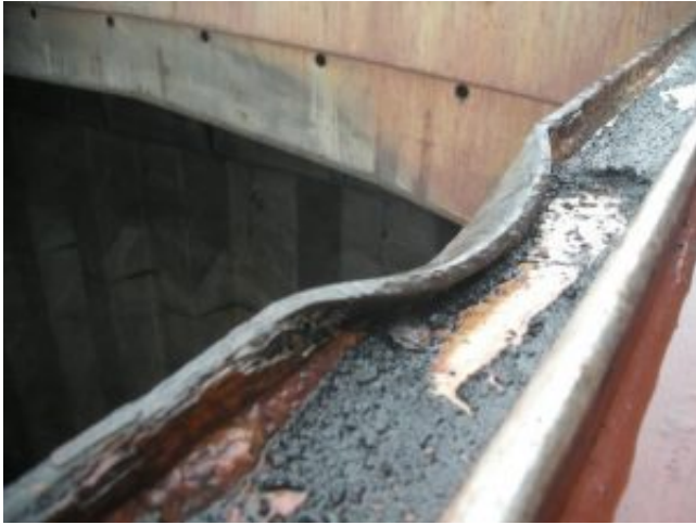
Figure 2: Damaged cargo hatch sill
