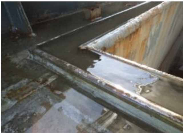
Figure 3: Overflowing drainage channels
